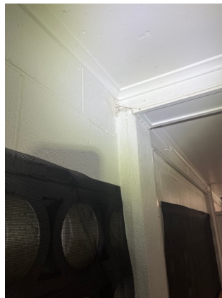
Image of no full termite shielding
