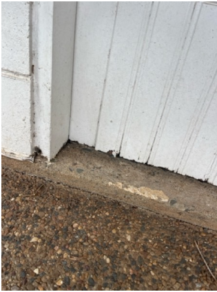
Image of fungal decay present in timber door frame and door.
