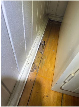
Image of old termite damage in timber flooring in bedroom 1
