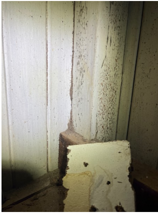
Image of old termite leads present on timber wall frame
