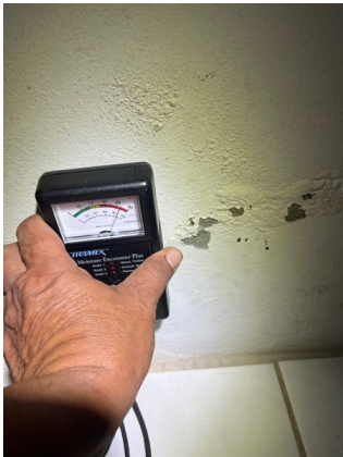
Image of high moisture reading observed in the enclosed subfloor wall
