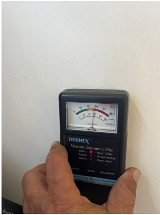
Image of high moisture reading observed in the wall of bedroom 3
