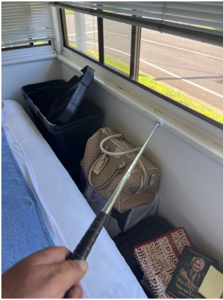
Image of timber window frame with old termite damage
