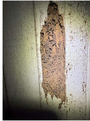
Image of Old termite damage present in timber wall
