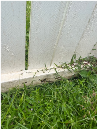
Image of fungal decay present in timber fencing
