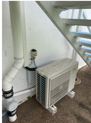
Image of aircon discharge next to the structure
