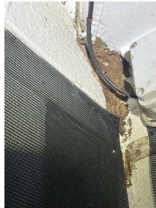
Image of old termite leads present on subfloor block wall and subfloor bearer
