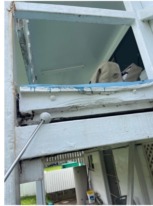
Image of fungal decay present in veranda timber
