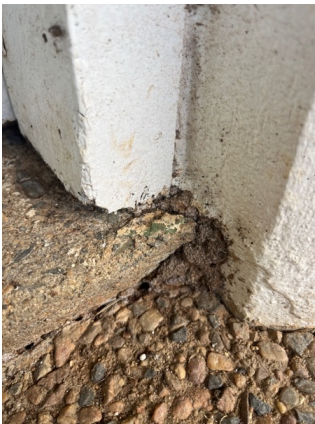
Image of old termite lead on the exterior concrete slab edge timber door frame.
