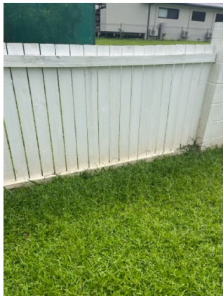
Image of timber fence in contact with the ground
