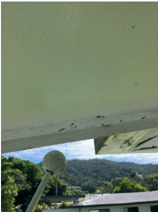
Image of fungal decay present in timber eave trim
