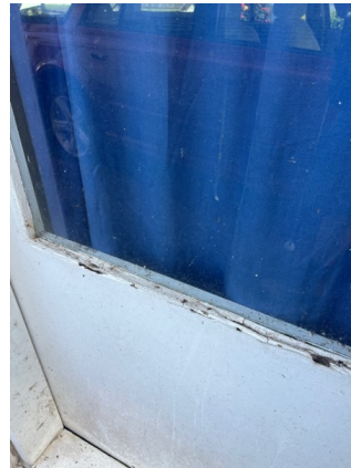
Image of fungal decay present in timber exterior door
