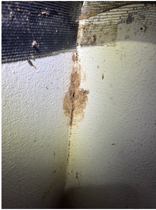
Image of old termite lead mark present on concrete block subfloor wall
